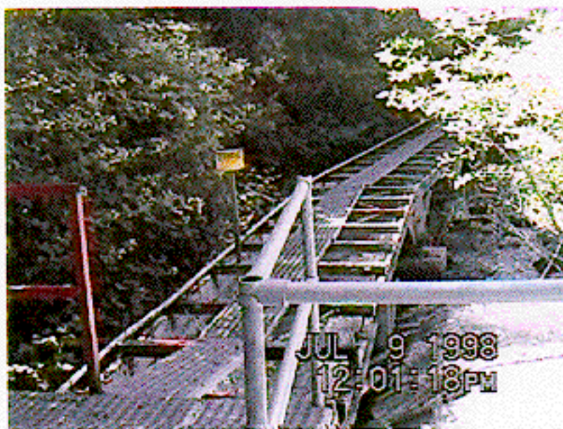
Photograph 10: Flume section of North Battle Creek Feeder, just downstream of Diversion. (credit DWR-ND)
