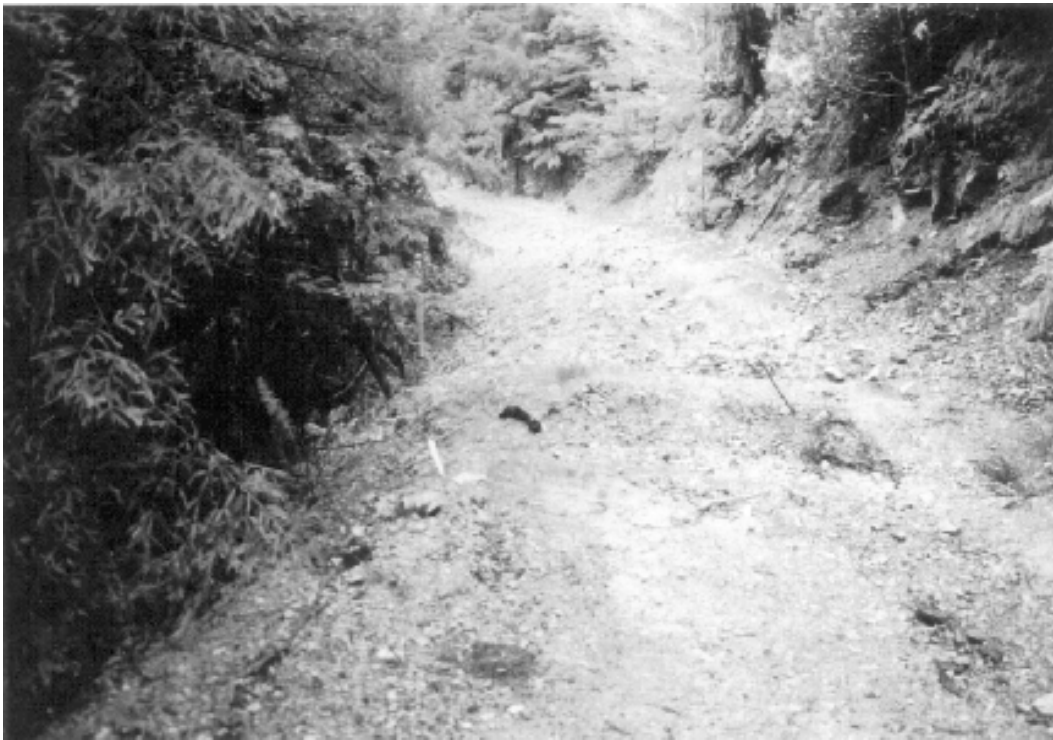
Figure 8. Site 94, G-005-01 Road. After treatment photograph from the same location. The unstable fill slope has been excavated beyond the orange flagging and the spoil material has been placed on the stable portion of the road bed with a prominent outslope. Note how the spoil material now extends to the base of the small conifer on the cutbank in the middle of the photo (the spoil material is nearly 3 feet deep at the former inboard edge of the road). A sizable cross-road drain has been constructed in the foreground of the photo to disperse road runoff.
