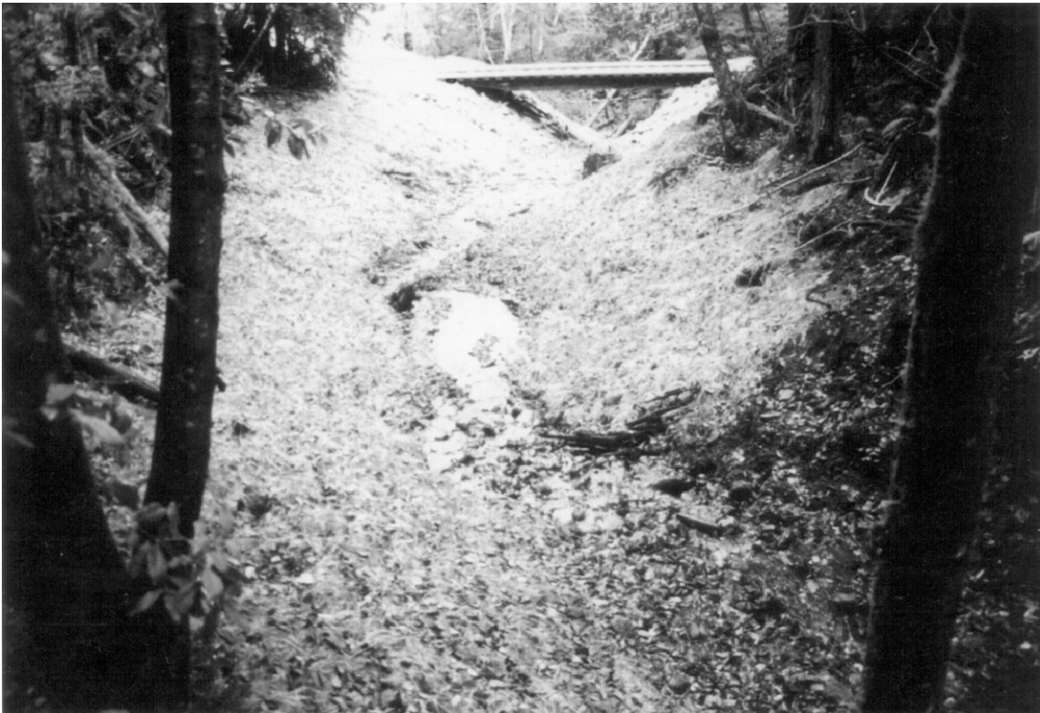
Figure 2. Site 50, G-006 Road. After photo looking downstream from the same location. All channel stored sediment and the culvert crossing have been excavated, and a flatcar bridge has been installed. The bridge was purchased with contributions from the MCRCD.
