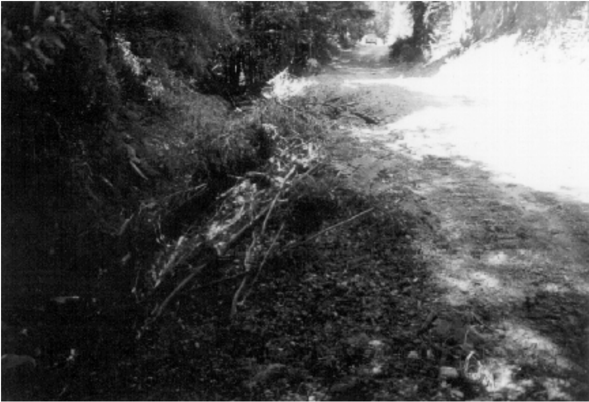
Figure 5. Site 13, B-Line. View upstream at the same reach of road seen in Figures 3 and 4. The truck in the distance is at the photo point where Figures 3 and 4 were taken. The natural stream channel flows toward the camera and is significantly constricted by introduced road fill and slash.
