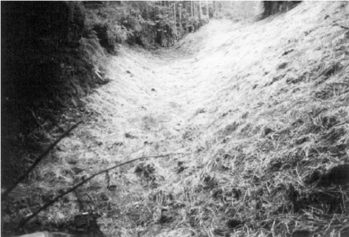
Figure 6. Site 13, B-Line. After treatment photo illustrating the application of in-place outslipping to remove a road. The natural stream channel has been reconstructed by removing all man introduced fill and slash, and now has a 6 foot wide channel bed designed to convey peak flood flows with minimal future erosion.
