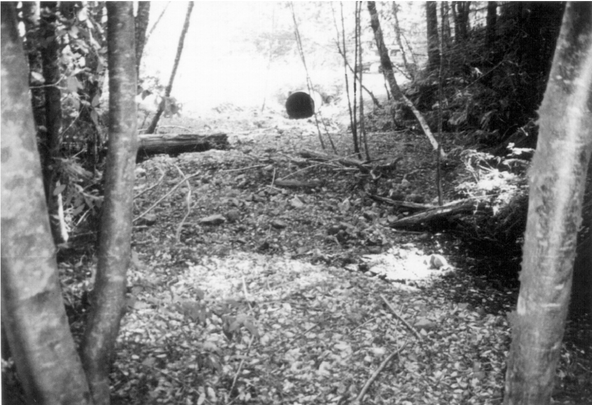
Figure 1. Site 50, G-006 Road. Before photo of site conditions looking downstream across large plain of channel stored sediment, with undersized 6 foot diameter culvert under the roadway.
