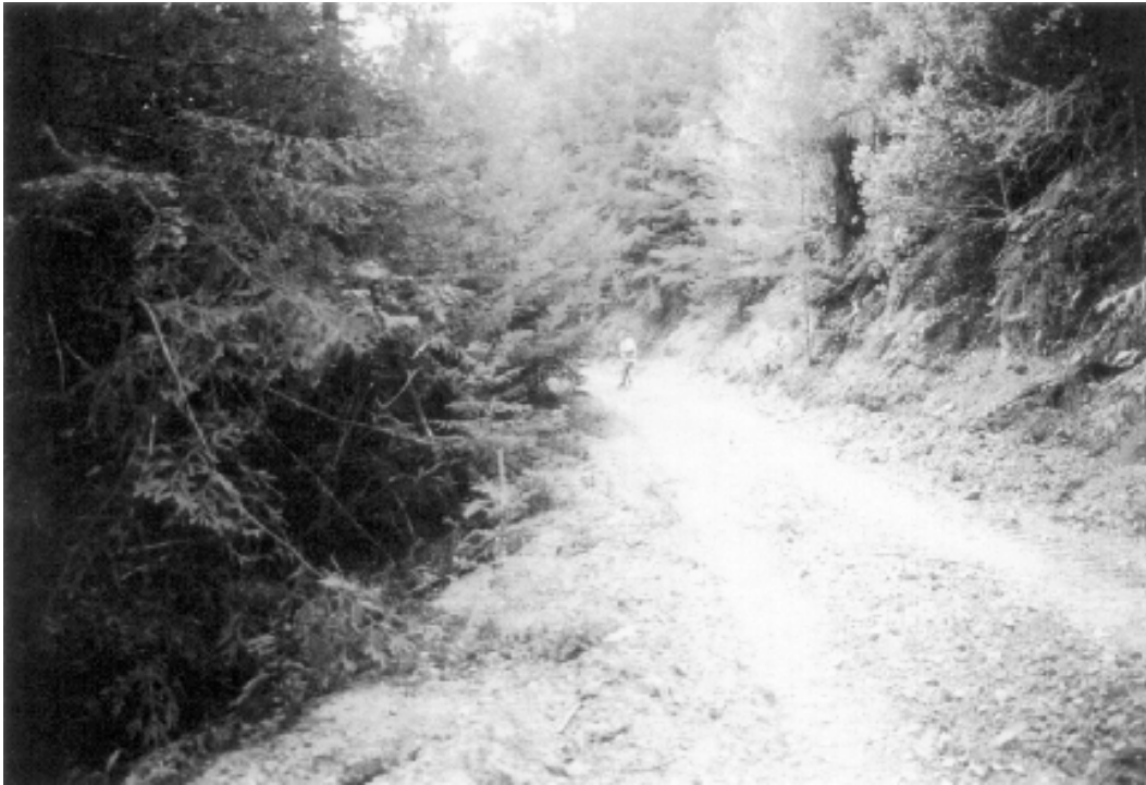
Figure 7. Site 94, G-005-01 Road. Before photo of road reach which exhibits unstable fill slopes between the orange flagging to beyond the person in the photo. A main fish bearing tributary to the South Fork Garcia is located 75 feet downslope of the road, and the potential fill failure was determined to have a risk of delivering some sediment to the stream.
