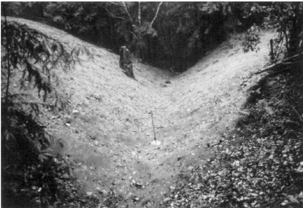
Figure 10. Site 100, G-005-01 Road. After treatment photo looking downstream. Note the orange flagging, redwood branch and leaf litter in the foreground denote the same location. The excavation involved removing over 900 yds 3 of fill from the stream crossing. The formerly buried stump helped to define the fill versus native soil material boundary. The channel has a 5 foot wide stream bed and 2:1 sideslopes designed to accommodate peak flood flows.
