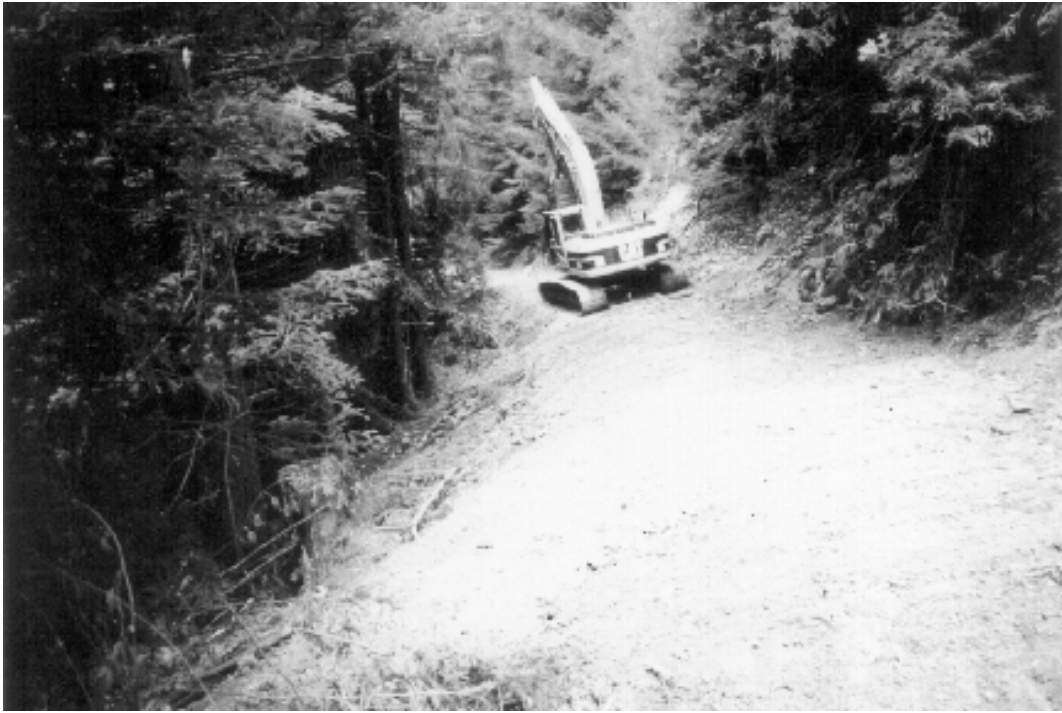
Figure 11. Site 99, G-005-01 Road. After photograph of section of road which has had unstable fill material excavated and placed with an outslope along the base of the cutbank (i.e. in place outsloping). The unstable fill, which posed a risk of sediment delivery to a downslope stream, extended out to the top of the stump prior to the excavation. This stretch of road was decommissioned.
