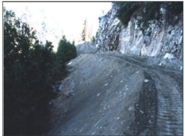
During imported fill disposal operations access to RX1 was maintained. Note the base of fill is at the outboard edge of the road.
