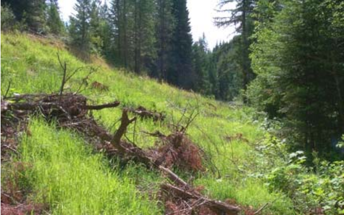
Recontoured portion of “old Road 416” adjacent to Quartz Creek. Note the use of slash and the successful revegetation of the slope.
