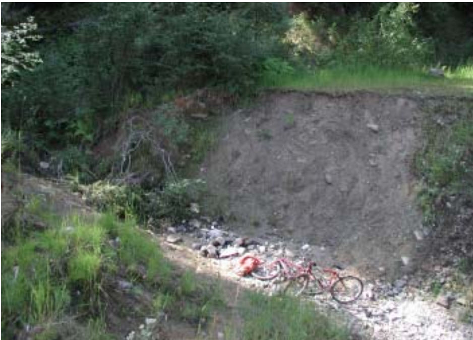
Fill Failure on Spread Creek at the Road 1013 Crossing. Note: the double culverts are still crushed and underneath the failure.
