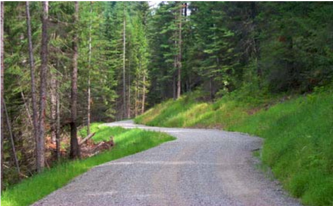
New construction of relocated Road 416. Note the stable lushly vegetated cut and fill slopes and the use of slash filter windrows.
