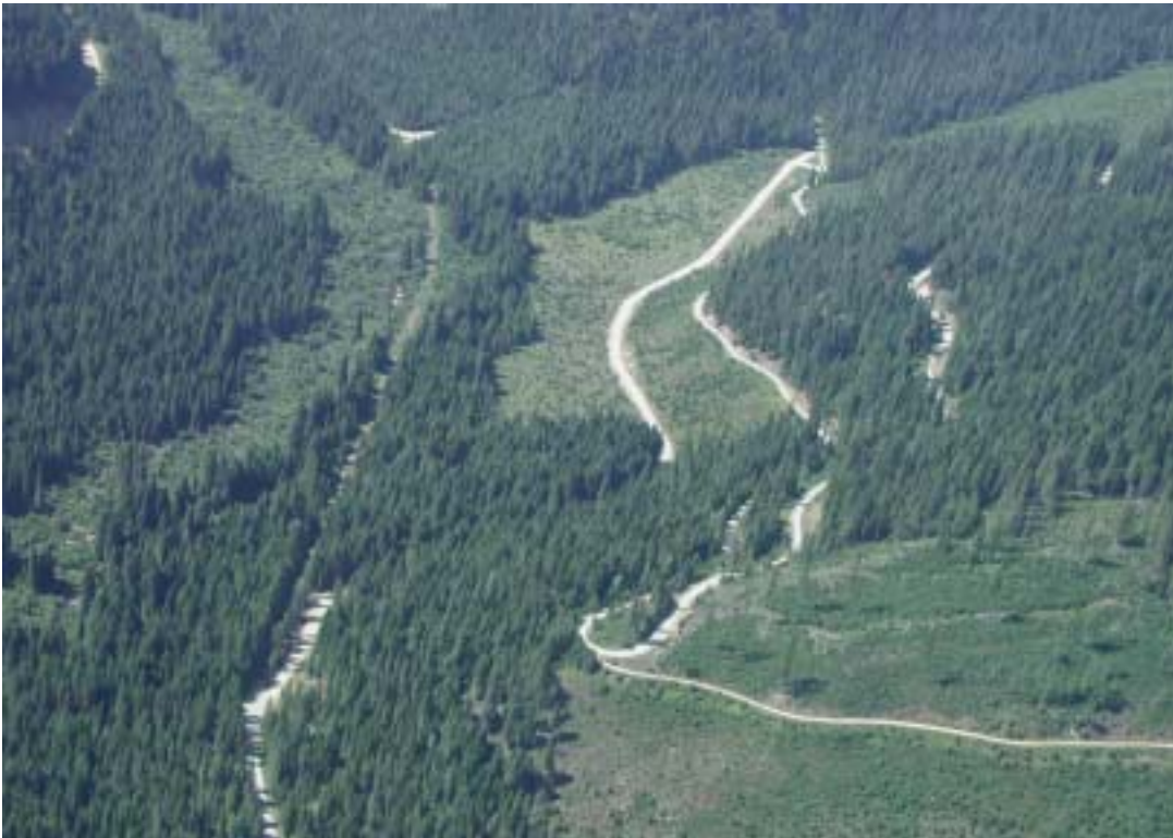
Photo showing reroute and obliteration of Road 312. Oblit. is linear feature on left. The new construction is the bright white road extending from the bottom left to the center.
