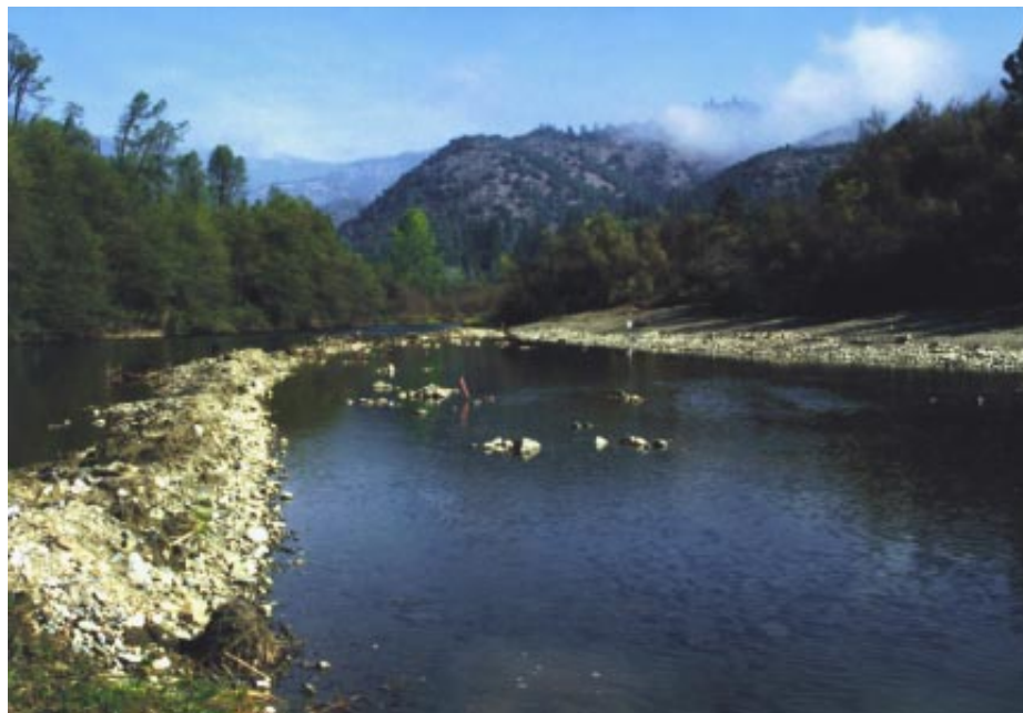
Figure 10.10 Sheridan Creek rehabilitation site. The long berm extending down the channel was a fine sediment retention berm used during construction and left intact after work was completed. The bank rehabilitation work can be seen along the upper right of the photo.
