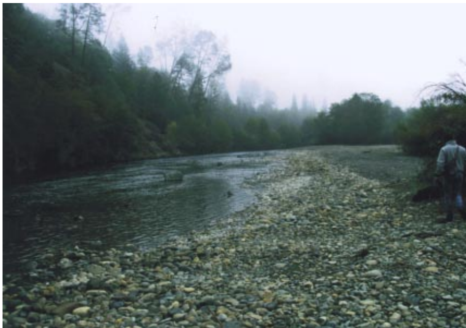
Figure 10.4 Bucktail rehabilitation site post-construction. Note boulder in the channel, left of center. Cobbles along constructed edge were placed as work was completed.
