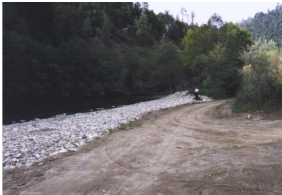
Figure 10.8 Post-construction bank at Steiner Flat. The riparian berm can be seen end-on behind the person in the photo. The cobbles that line the bank were artificially placed during construction.
